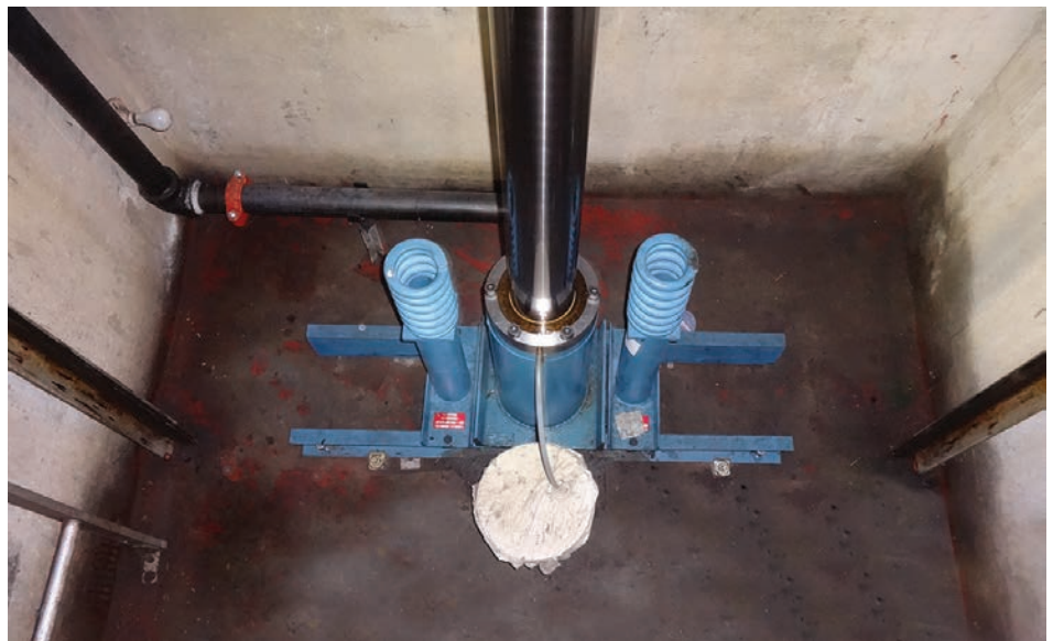
Hydraulic Elevator Pit
