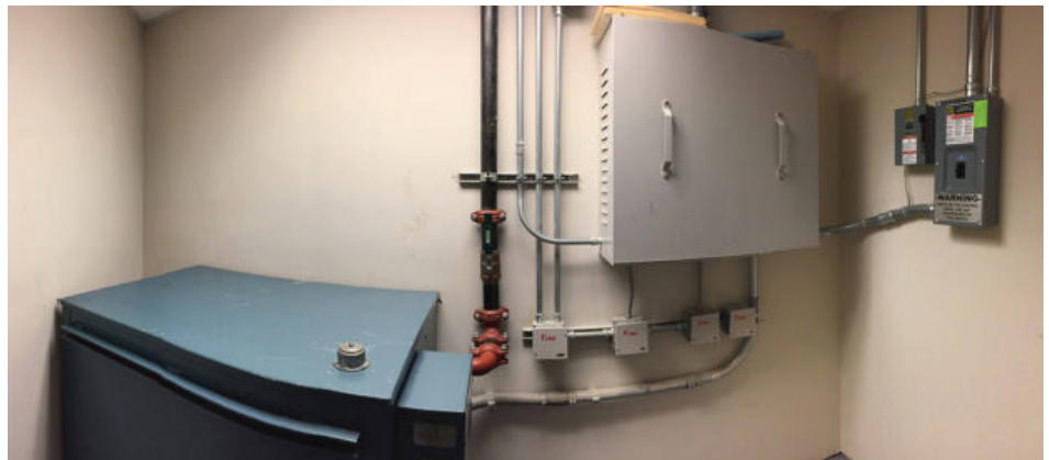
Elevator Machine Room of a DC Elevator Client
