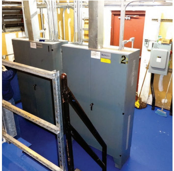
Machine Room After Modernization
