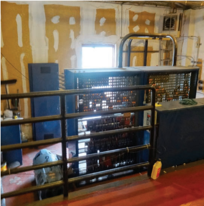
Machine Room Before Modernization
