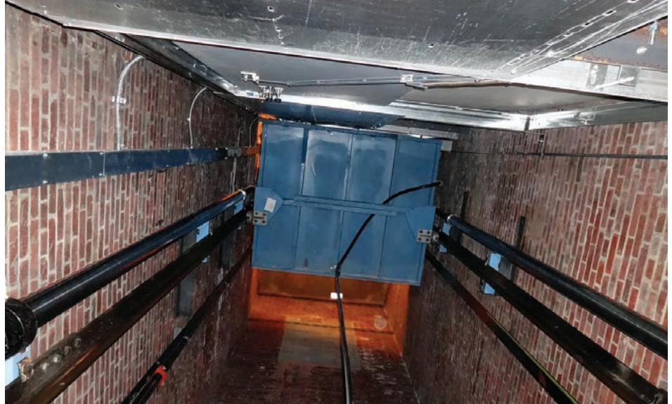
Hydraulic Elevator Hoistway
