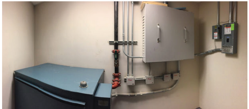
Elevator Machine Room of a DC Elevator Client
