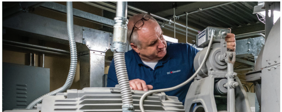
DC Elevator Technician Inspecting an Elevator Motor
