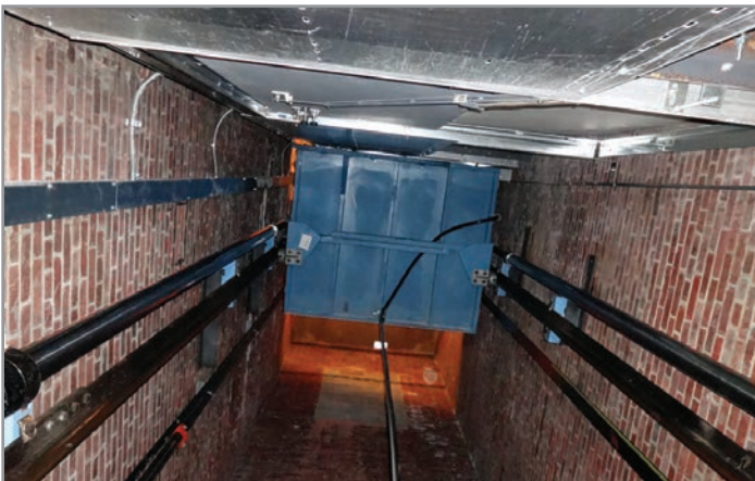
Hoistway of a Hydraulic Elevator
